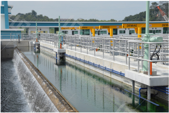
LANGAT 2 WATER TREATMENT PLANT , HULU LANGAT
